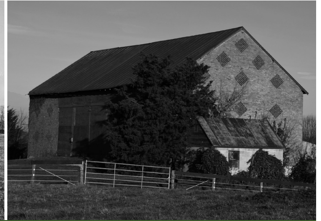
The Jacob Homar Barn, built in 1832, is one of only two remaining brick bank barns in Jefferson County.
