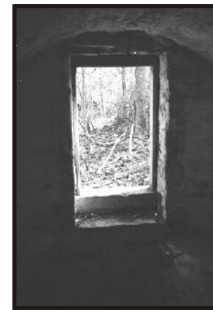
Figure A-16. Bath House, closeup of left wall and window (as you face the Shenandoah River). Doorway on opposite side is visible. Bill Theriault, Photographer, 1997.
