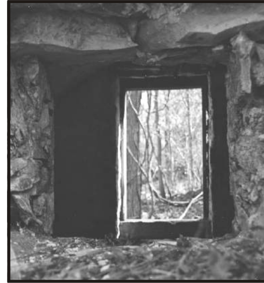
Figure A-14. Bath House, closeup of left wall and window (as you face the Shenandoah River). Doorway on opposite side is visible. Bill Theriault, Photographer, 1997.
