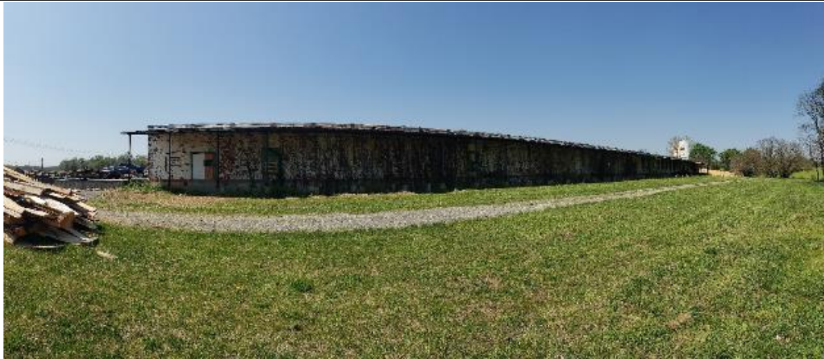
Image 9. Southeast side of the building (which faces the railroad tracks) from south corner.
