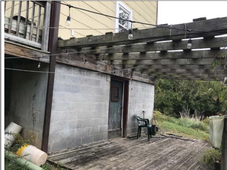
WV_Jefferson_County_Susan Thornton House_0007 Susan Thornton house cellar addition. View southwest to northeast.
